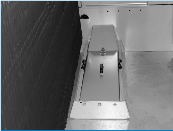
Cold water basin and basin strainer
