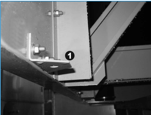
Inside view plenum section
