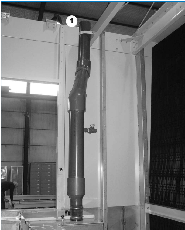
Pump piping lower section
